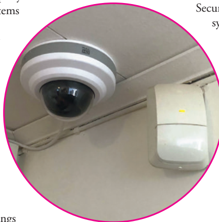
Martin Bäckman also emphasises that security cameras are now also commonly part of new home security system installations.
