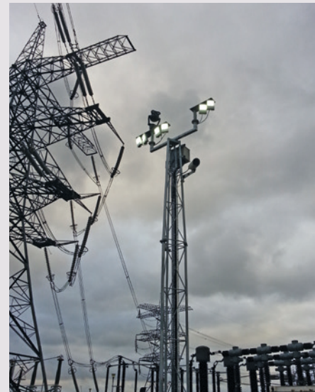
Perimeter surveillance installation with Vario2 white-light illuminators from Raytec.
