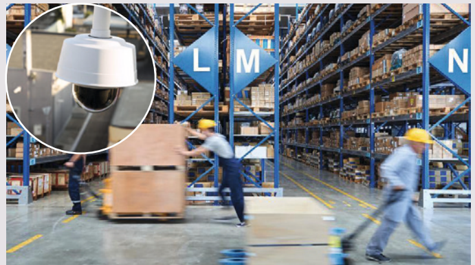
Inside the warehouse, cameras are positioned above giant roller-shutters for an ideal perspective of the main floor while also monitoring passage through the main access points.
