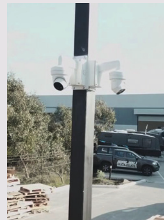
Ten 4K-resolution Acusense Live Guard cameras are installed around the property.
