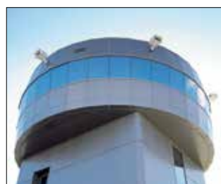
The cameras of the Panomera system for this airfield project were installed at a considerable height, close to the roof of the Apron tower.
